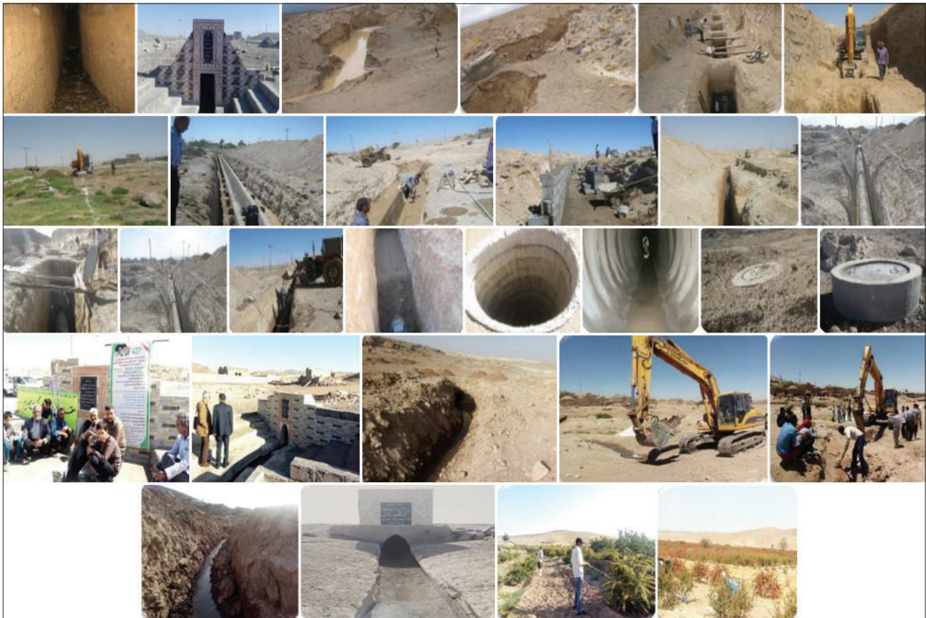
Figure 4: Various phases of Koling, installing Kol, repairing and reconstructing of aqueducts (qanats) repairing and reconstructing in Salamabad Aqueduct Village and other queducts (qanats) in rural regions in the South Khorasan Province in east of Iran. Plus cultivating Barberry shrubs ( Berberis vulgaris ) that are drought resistant plants and favorable for dried conditions of this region. (two last pictures) (pictures by author, 2015–2021) [8]
